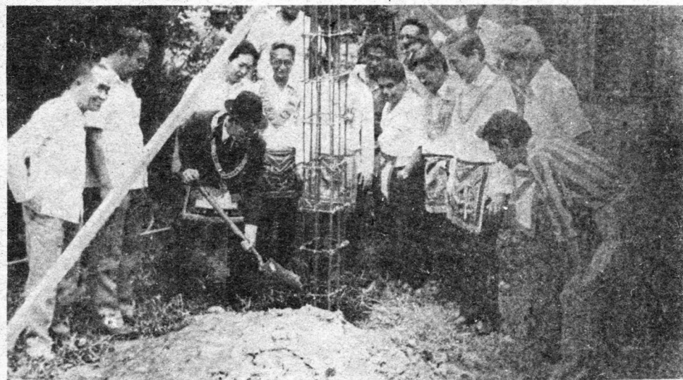
1st pouring concrete for the Temple building of Tumaui Lodge No. 25. August 5, 1988, Isabela.
