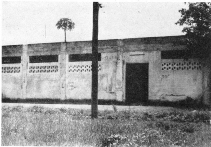
Temple of Bataan Lodge No. 104 in Orani, Bataan. It is undergoing renovation due to the damage caused by recent typhoons.
